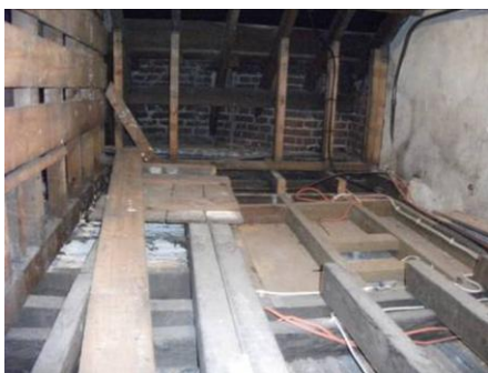
Picture of void in apartment at Hampton Court
