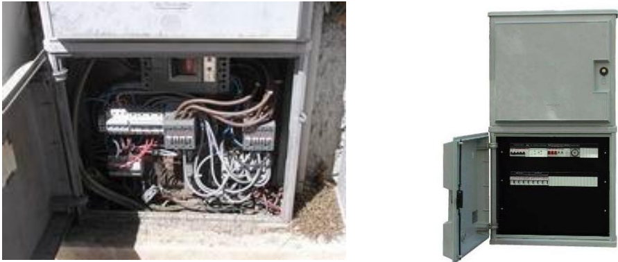
Figure 1. Renewed or new electrical boards
