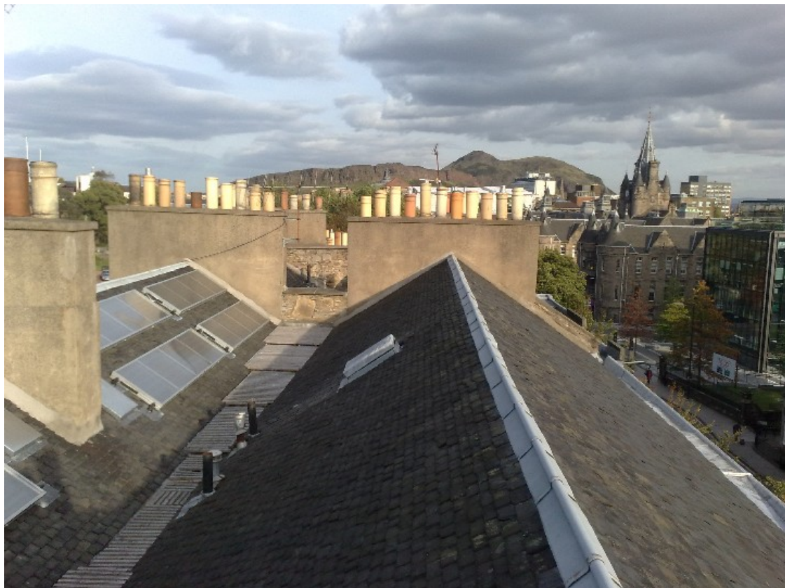
Solar systems installed in the hidden roof valleys of listed Georgian buildings (© Changeworks)
