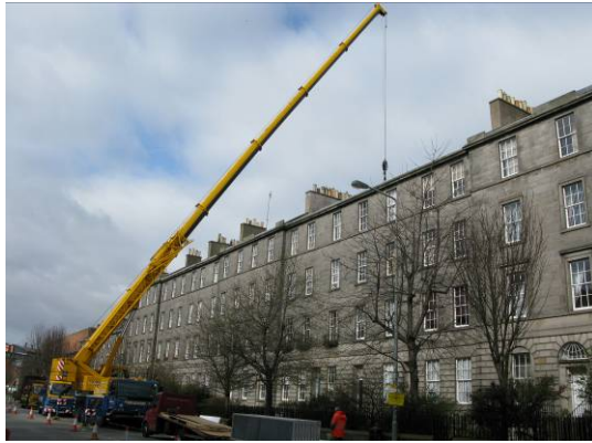
The solar panels being delivered onto the tenement roofs (© Lister Housing Co-operative)
