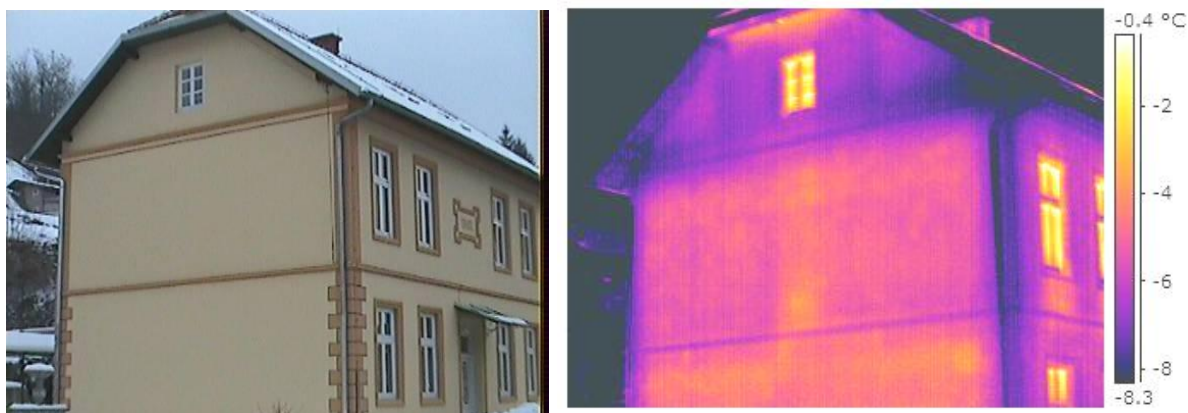
Figure 2. Photography and thermogram of a building in Duga Resa
